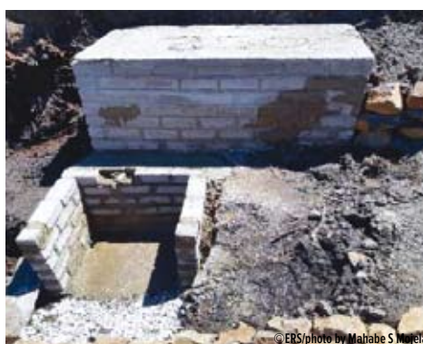
Above - A formal collection chamber sits behind the access point where water can be collected from the tap.
